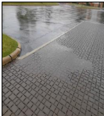
Surface ponding over PICP indicating clogged joints and the need for maintenance. Credit: Chagrin River Watershed Partners, Inc.
