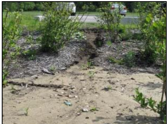
Erosion of side slopes and subsequent sediment accumulation within bioretention area and contribute to clogging issues. Credit: Summit Soil & Water Conservation District
