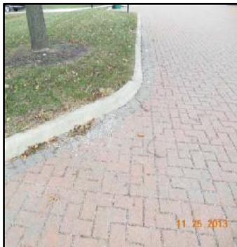
Permeable interlocking concrete pavement (PICP) shown with accumulated sediment along the curb indicating need for maintenance. Credit: Chagrin River Watershed Partners, Inc.
