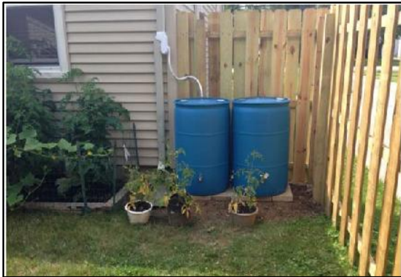
Dual rain barrels connected in series from the downspout diverter. Once barrels are full, rainwater continues down the downspout. Credit: Chagrin River Watershed Partners, Inc.
