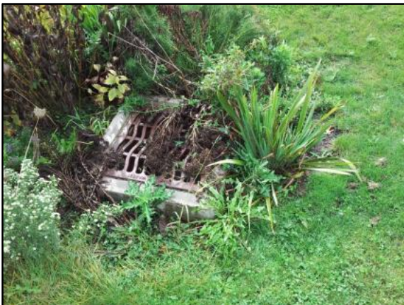
Stormwater flow will be blocked by the dead vegetation on the outlet catch basin grate . Credit: Chagrin River Watershed Partners
